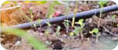
STP treated water for gardening
